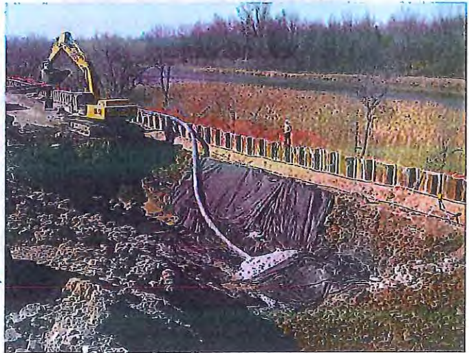
▶ Installed Water Barrier Groundwater Containment Wall (sheet piles) and the installation of the leachate interceptor trench
