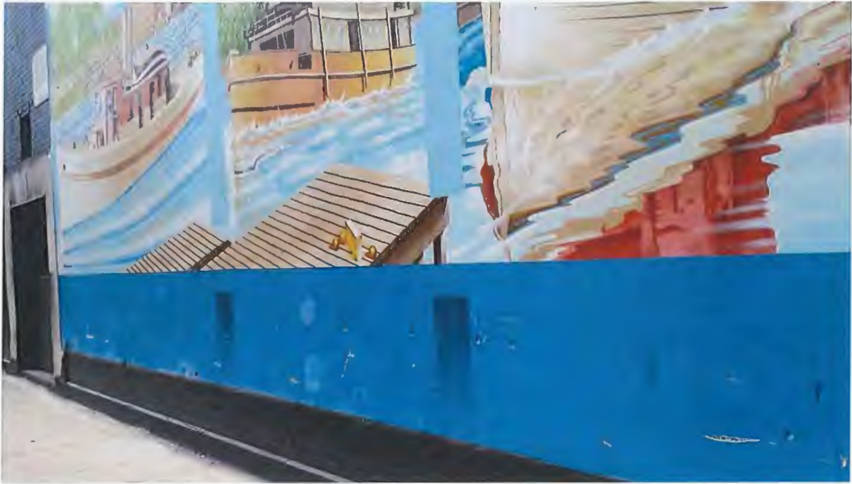
Figure 7 Damage on lower left side of mural. Photo: N. Reid
