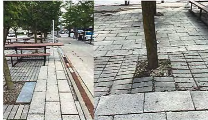
Safety - Paving/Drainage Require Repairs
