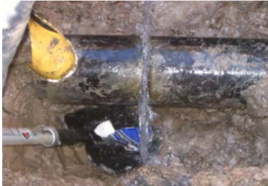
Figure D-1: Circumferential watermain break with flow maintained until after an Air Gap was established.
