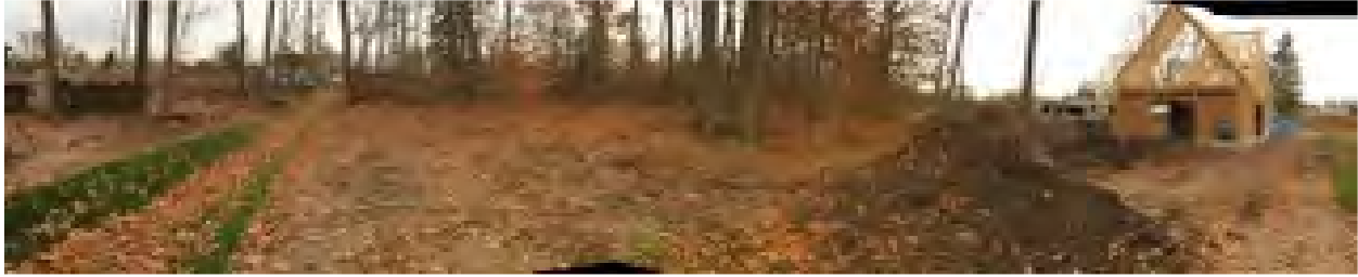
Photo 3. A new east-west drainage ditch along private woods increasing potential for the drainage of the upland woods first observed in Nov 2019.
