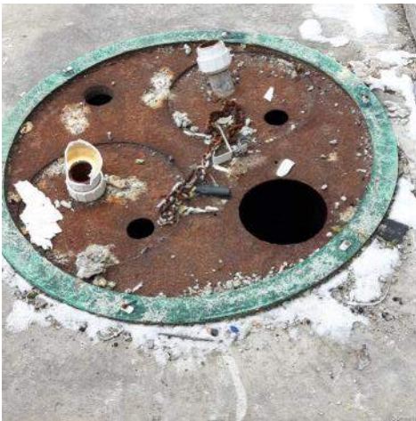
Photo 9: View of UST south of Site Building-Y.
